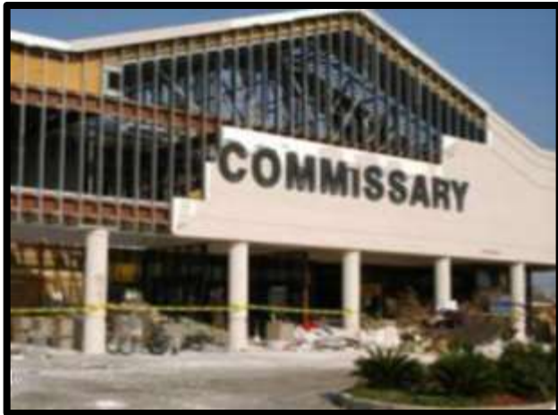
Damage to Naval Construction Battalion Center (NCBC) Gulfport Commissary caused by Hurricane Katrina in September, 2005.
